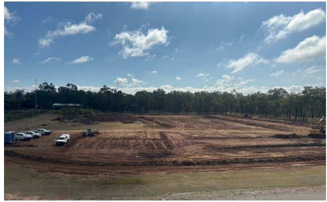
Figure 13: Earthworks recently commenced on Stage 2 of the HPA First Project (below image is as of 15 th August 2024)
