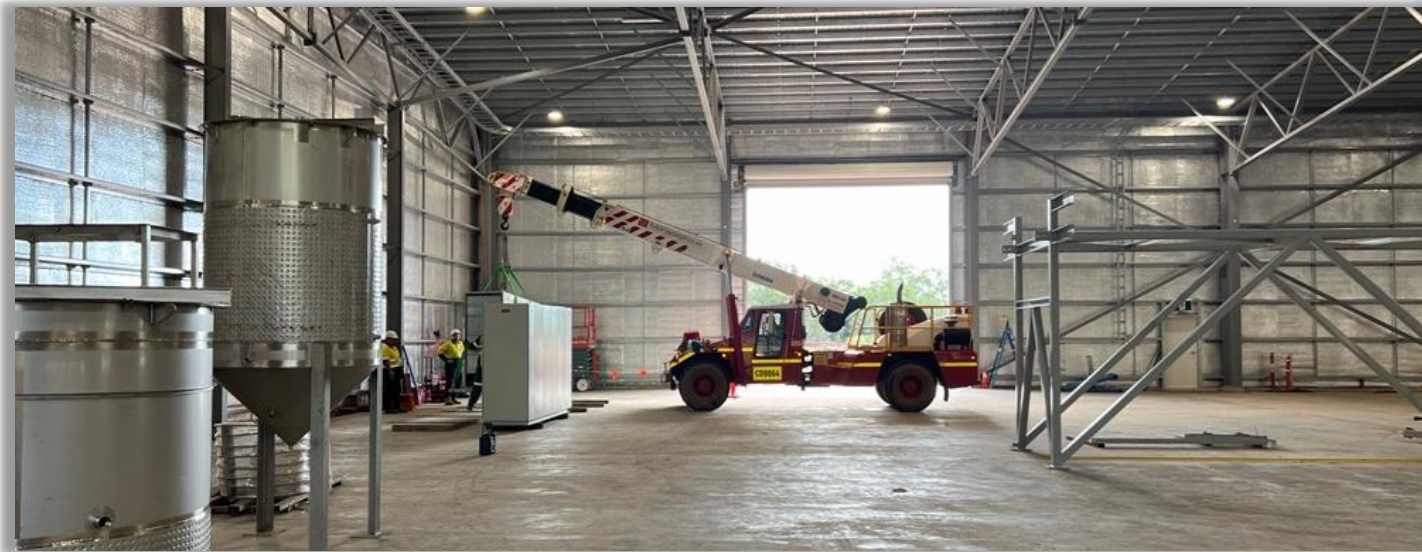
PPF Building Interior - Lighting installed and energised, with process equipment deliveries continuing
