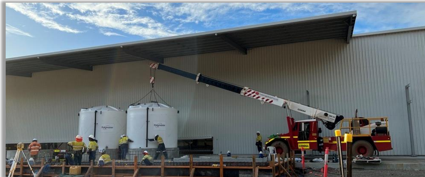
Installation of PPF reagent tanks
