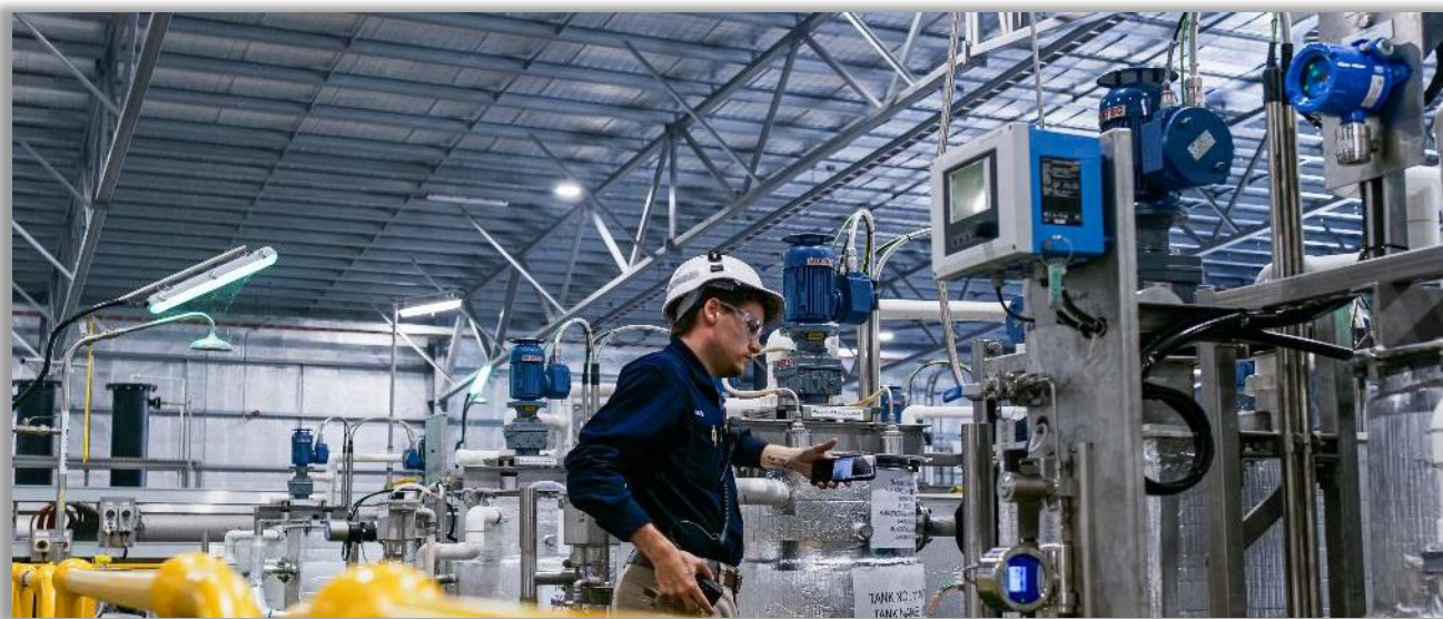
Aluminium Solvent Extraction (SX) Circuit – Stage 1 PPF
