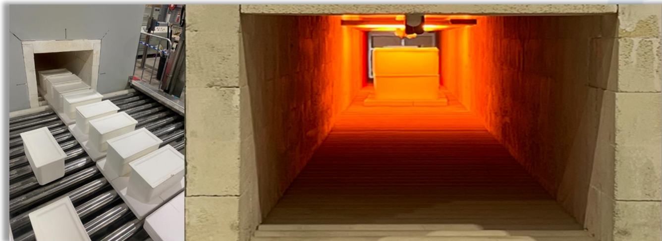
HPA tunnel kiln – in final commissioning
