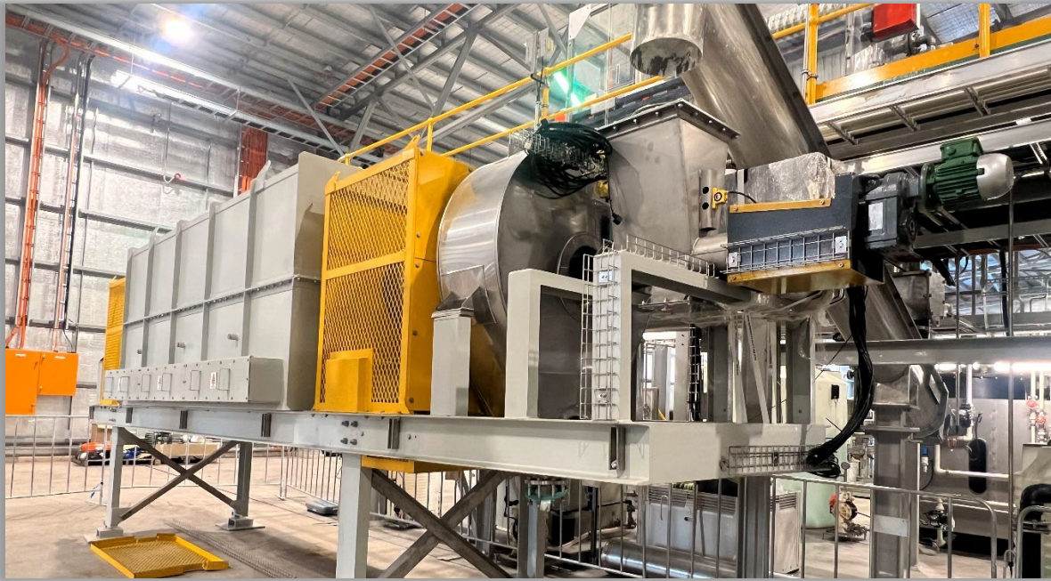
HPA dryer installed into Stage 1
