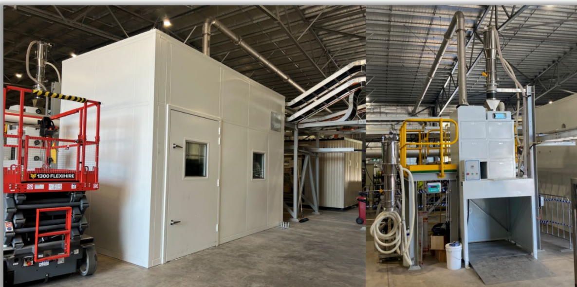
Jet mill enclosure (LHS) and HPA rolls crusher (RHS) installed
