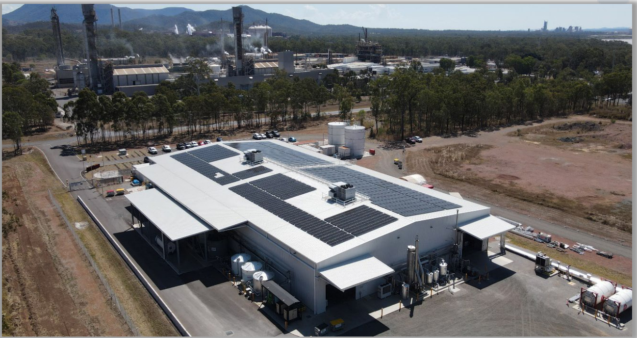
Stage 1 PPF – showing completed rooftop solar installation
