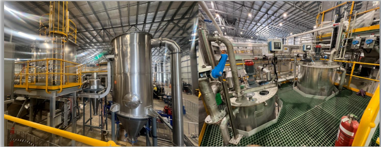
Area 1270 (high-purity boehmite and alumina trihydrate) circuit – under commissioning. Spray drier on LHS
