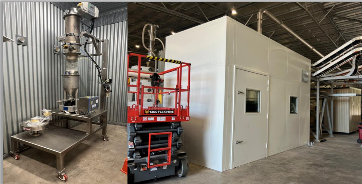
Jet mill unit (LHS) installed into the soundproof enclosure (RHS)
