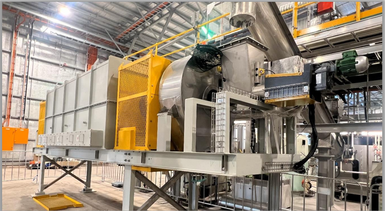
HPA dryer installed into Stage 1 and under commissioning
