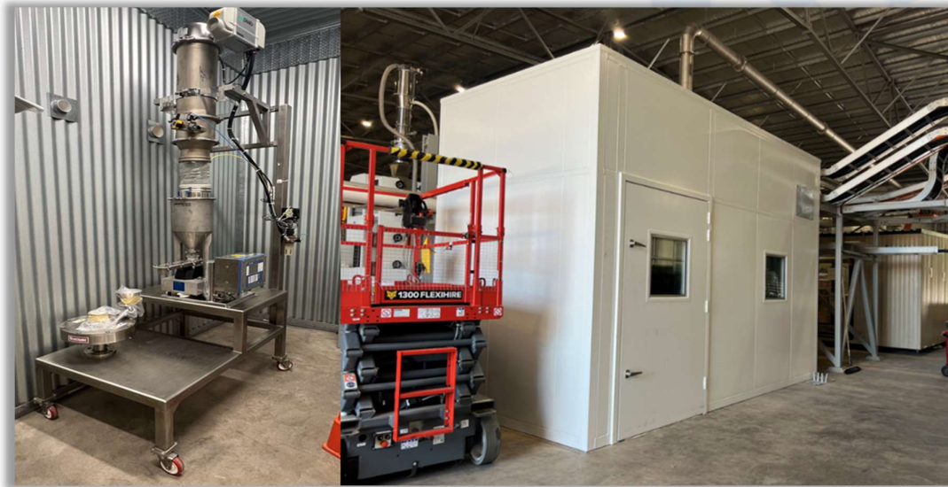
Jet mill unit (LHS) installed into the soundproof enclosure (RHS)
