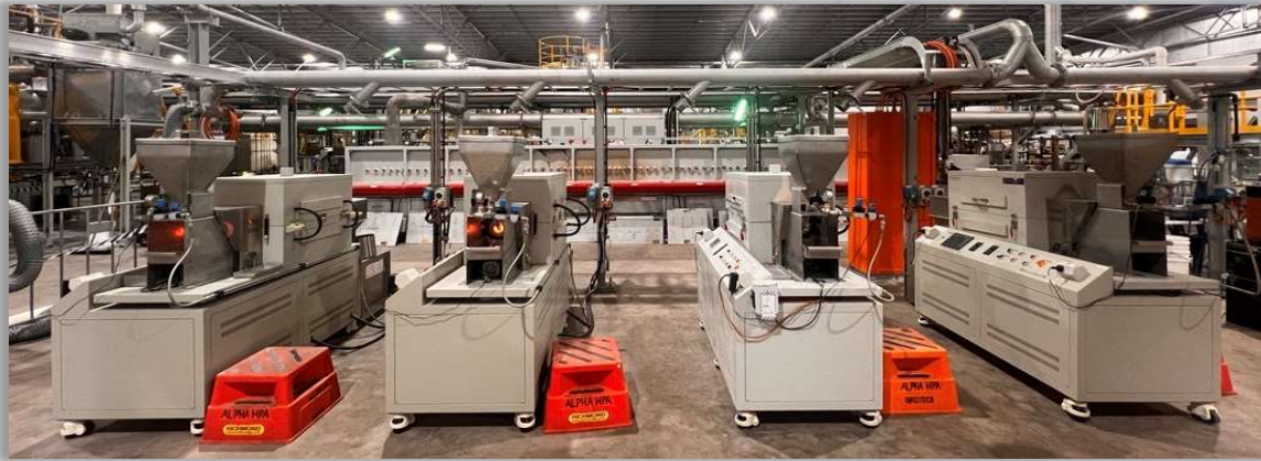
HPA rotary kilns – in final commissioning
