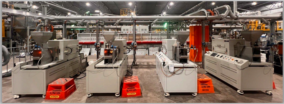
HPA rotary kilns – in final commissioning
