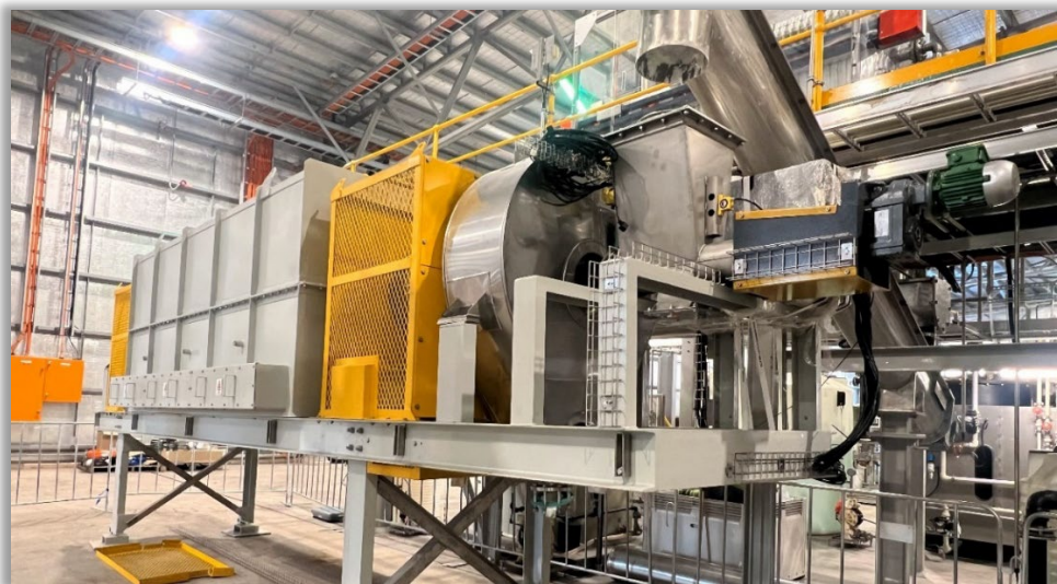
HPA dryer installed into Stage 1 and in commissioning
