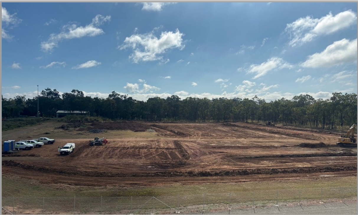
Earthworks commencing on Stage 2 of the HPA First Project – 15 th August 2024 (Looking North – taken from roof of Stage 1)
