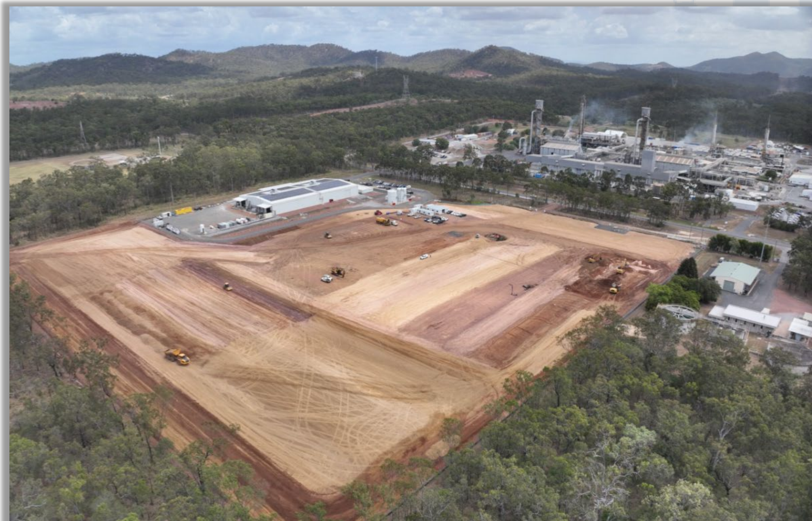
HPA First Project site looking southwest, showing earthworks well advanced, Stage 1 PPF and Orica Yarwun to the right of picture.
