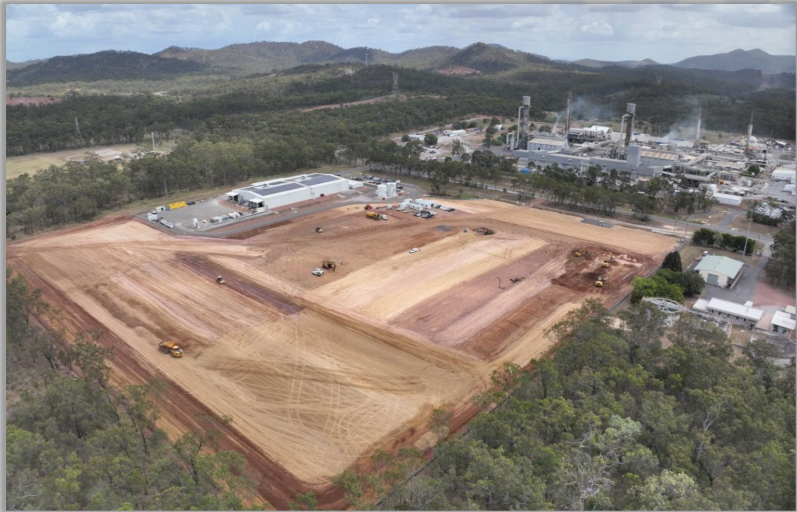
HPA First Project site showing earthworks well advanced, Stage 1 PPF and Orica Yarwun to the right of picture.
