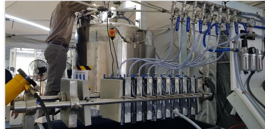
Pilot Plant – HPA Pre-cursor Circuit
