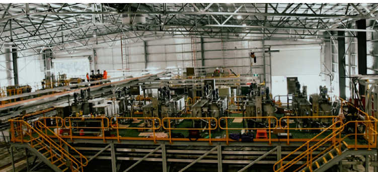
► Completed mechanical installation of solvent extraction (SX) circuits
