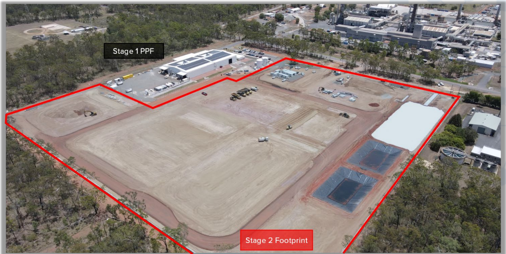
HPA First Project site looking southwest, showing earthworks near completion. Orica Yarwun to the top right of picture, lined retention ponds to the right of picture.
