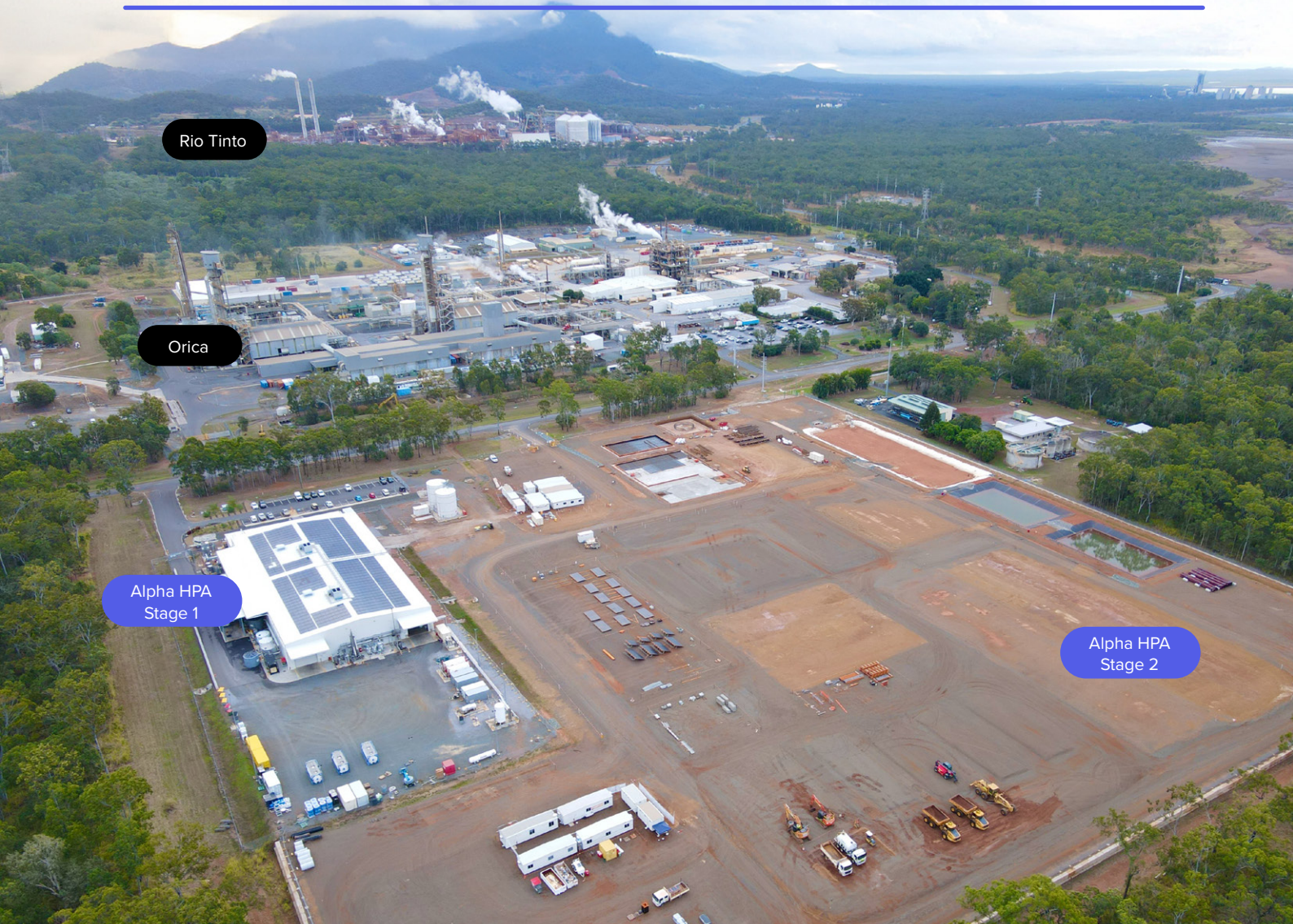
HPA First Project site looking west, showing completed earthworks and commencement of civil works Orica Yarwun in midground and Rio Tinto Yarwun alumina in background
