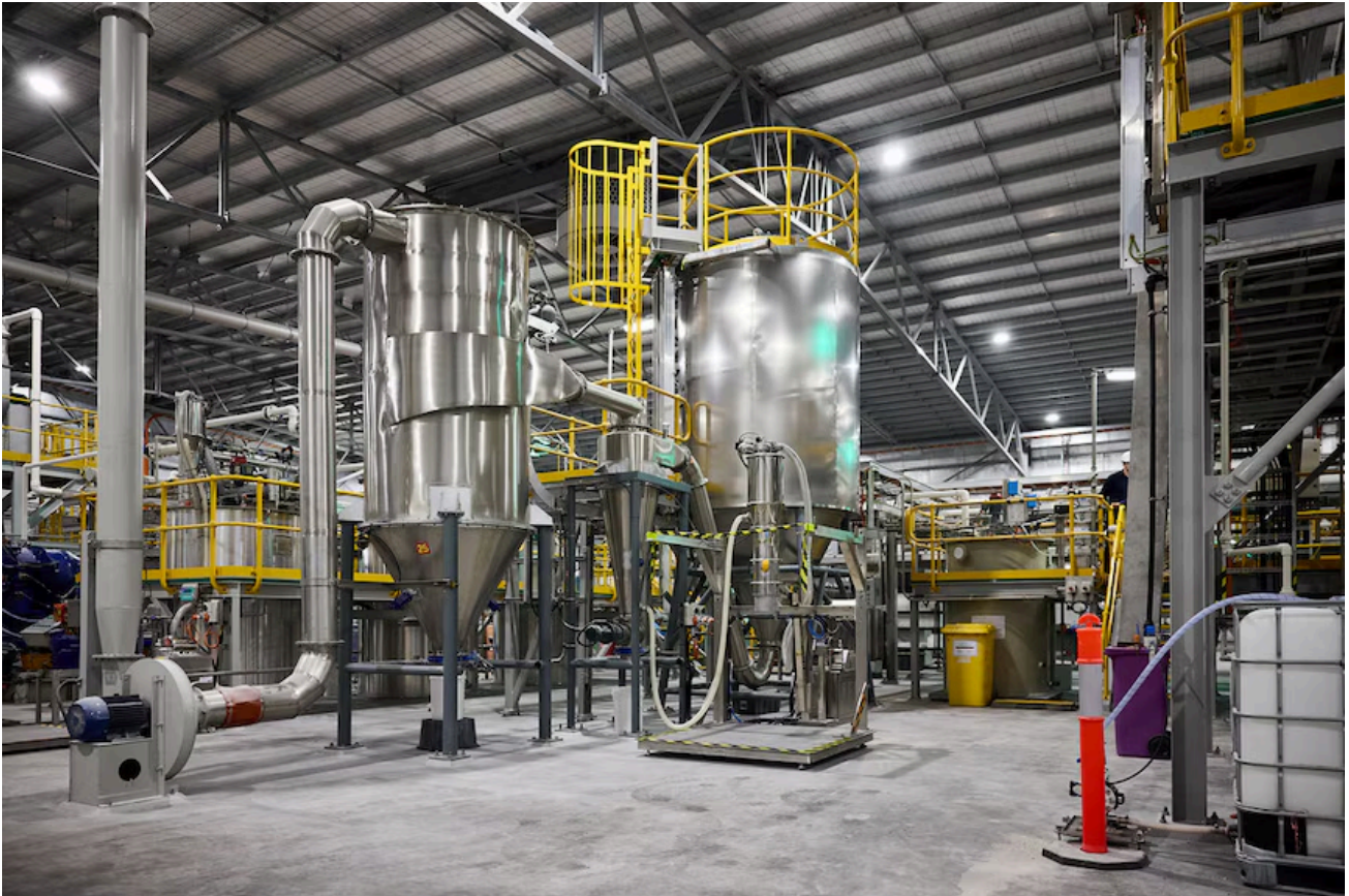
The interior of Alpha HPA's stage one facility in Gladstone. (Supplied: Alpha HPA)
