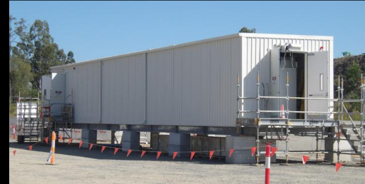
Pre-Assembled Electrical Switchroom
