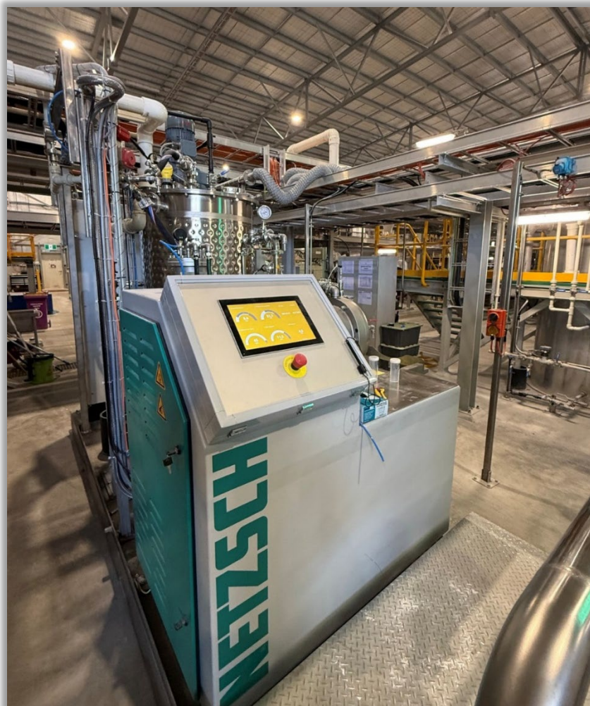
Fully installed alumina nano mill – within the Stage 1 Facility
